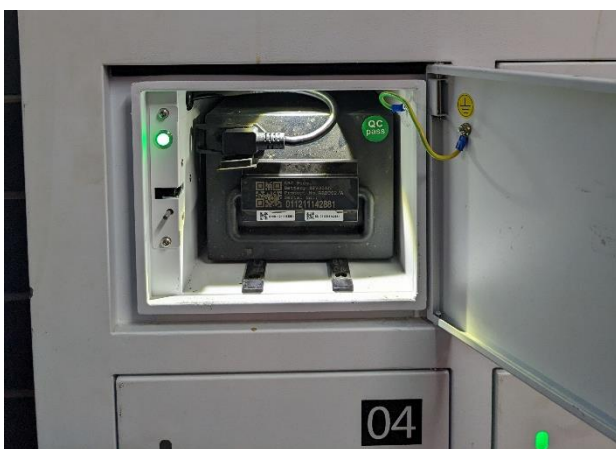
Figure 18. An automated battery swapping cabinet by Arc Ride in Nairobi, Kenya. Photo credit: Tom Courtright.
