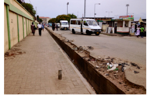
Uncovered drains along many streets
